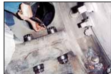
Split gear segment on rotary kiln.
